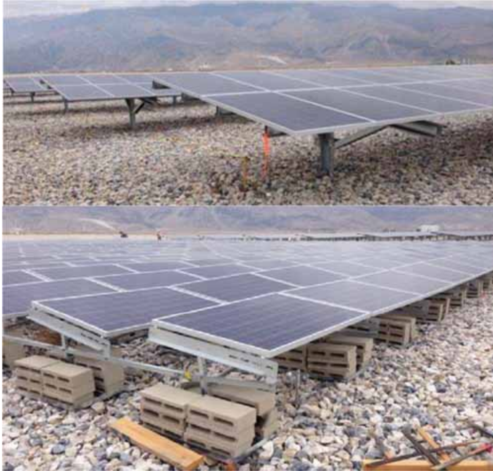
FIGURE 4-14 Solar panel testing installed on gravel at Owens Lake using pile-driven mounts (top) and squat ballast mounts (bottom). SOURCE: Schaaf, 2019.
