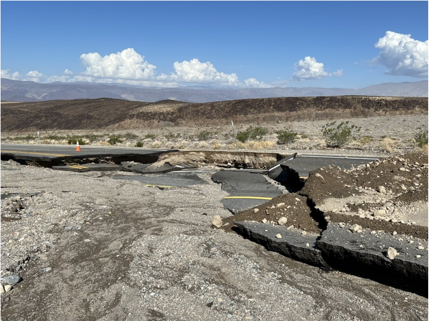
Flash flooding on September 10, 2022 caused extensive pavement damage on CA-190.
