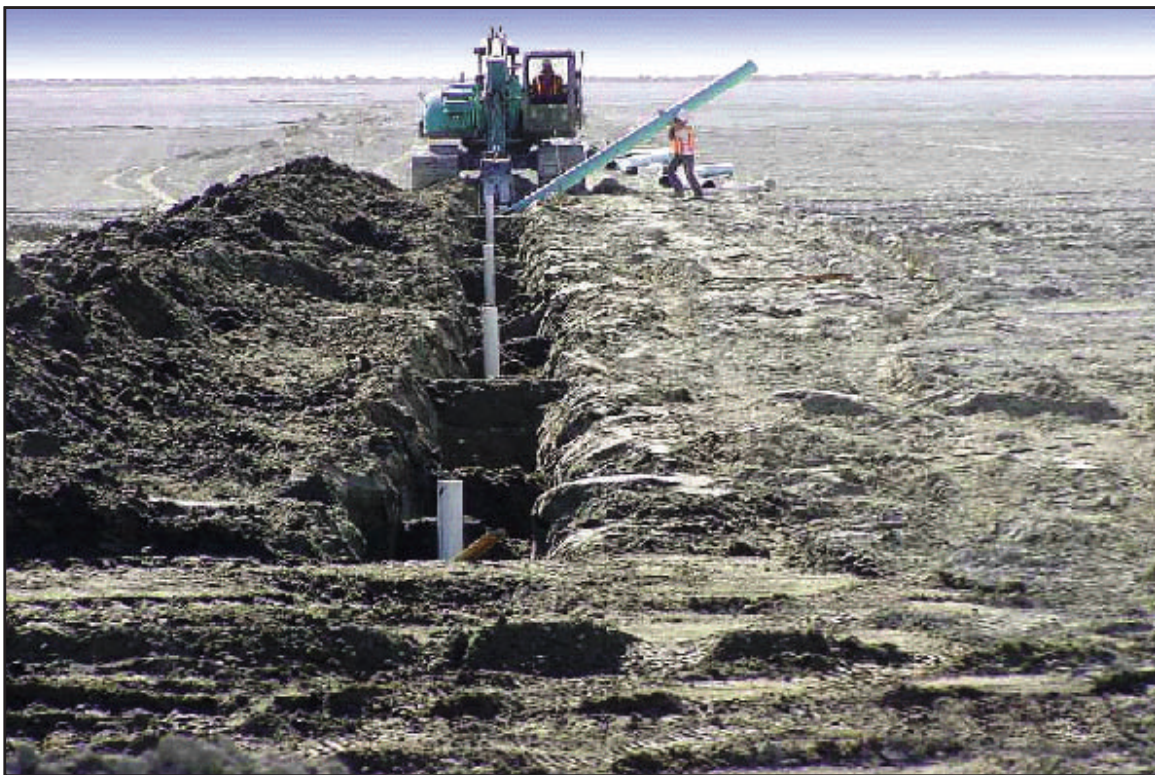
Field Irrigation Lines
