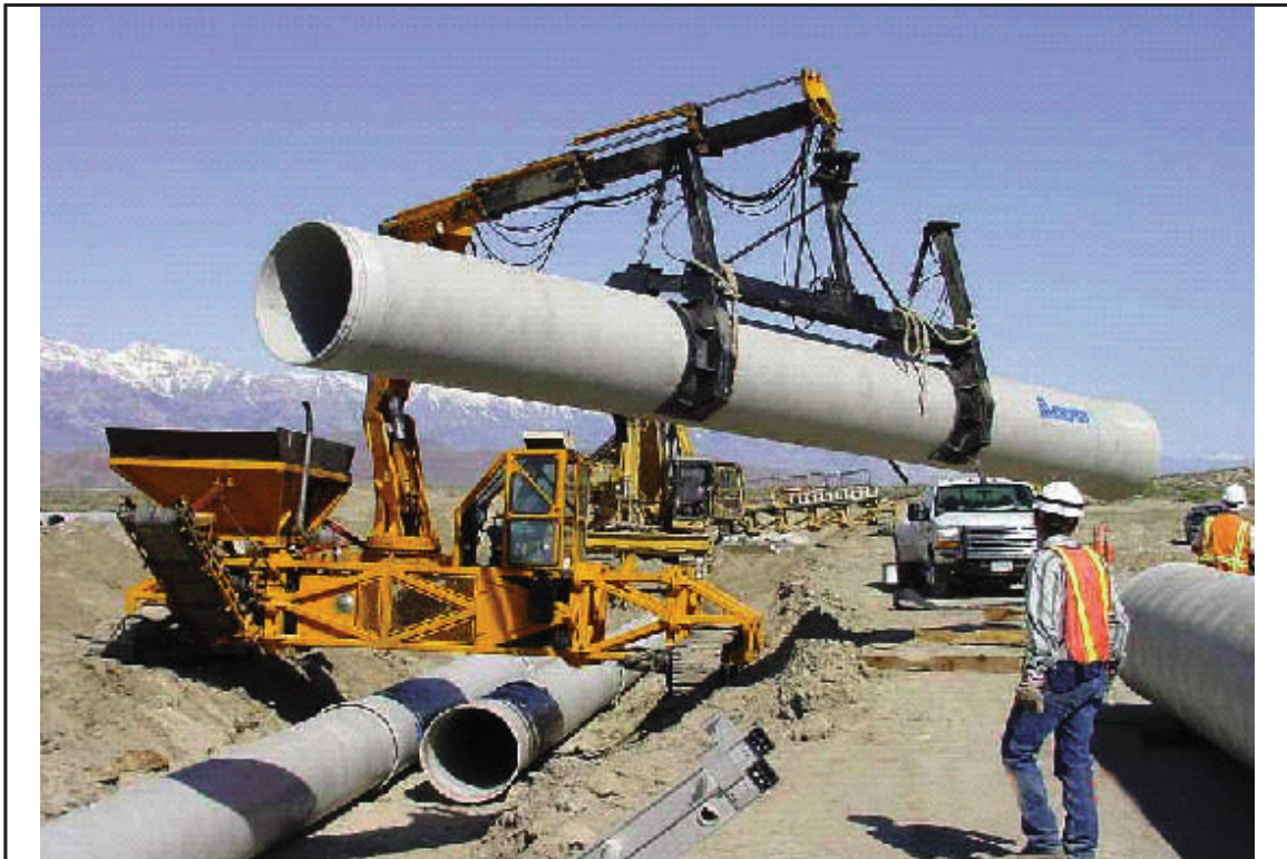
Water Supply Mainline
