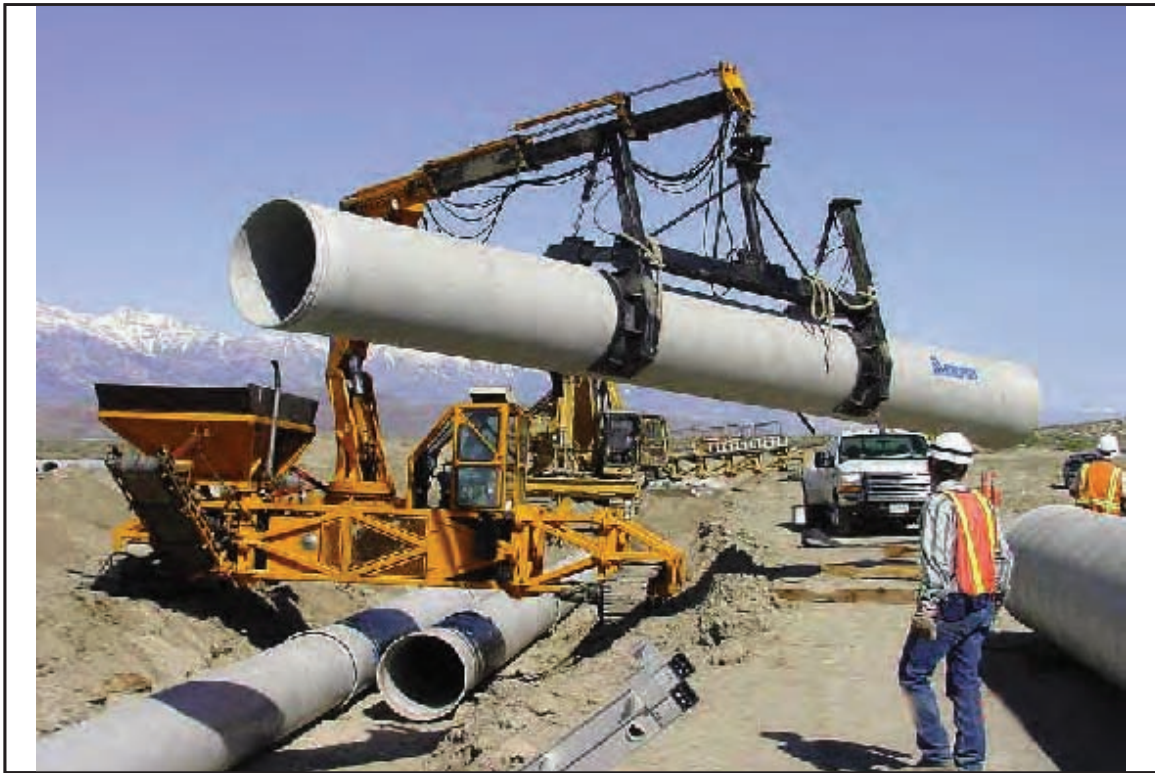
Water Supply Mainline
