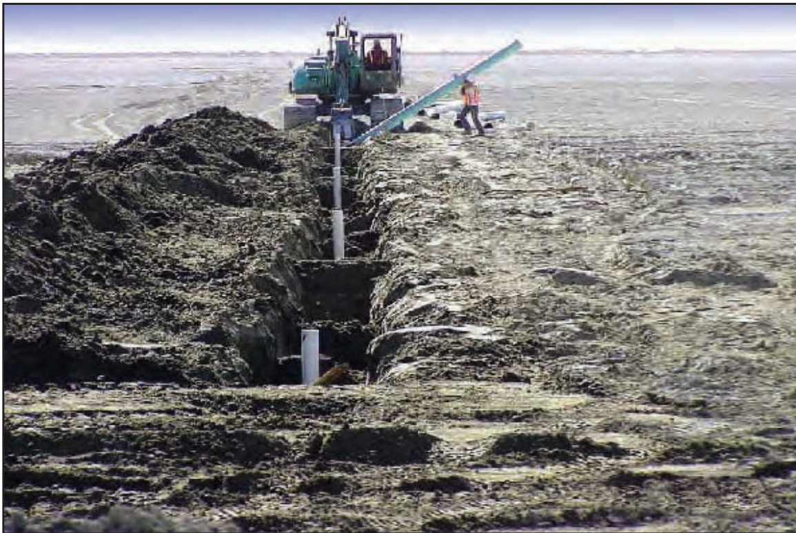
Field Irrigation Lines
