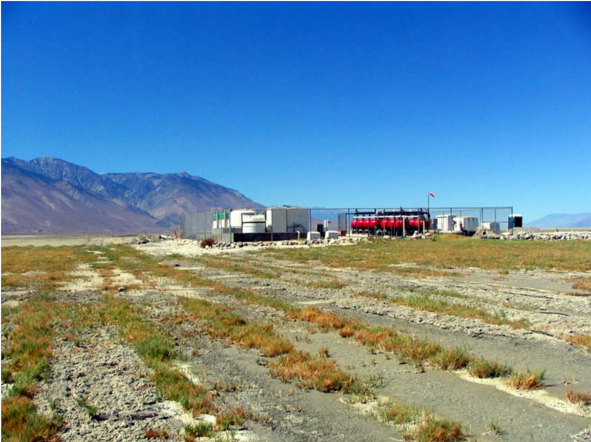
Figure 5.15b – Managed Vegetation – equipment pad with sand filters and chemical tanks
