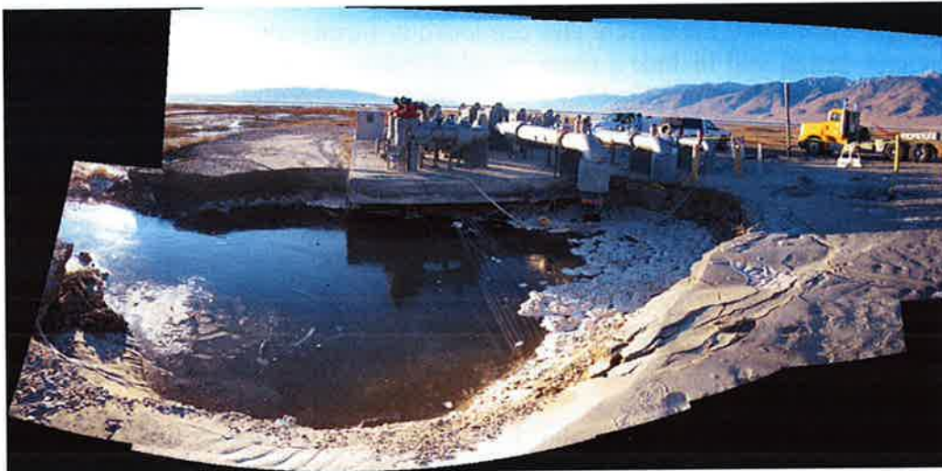
Photo 1: View of Damage Looking South
