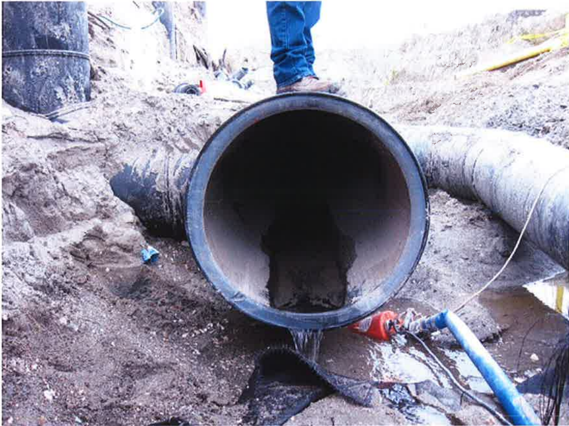
Photo 3: View of the damaged 30 inch pipe without end cap with water removed looking West.
