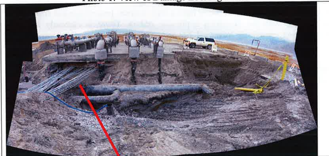
Photo 2: View of Damage Looking South after dry down and excavation.
